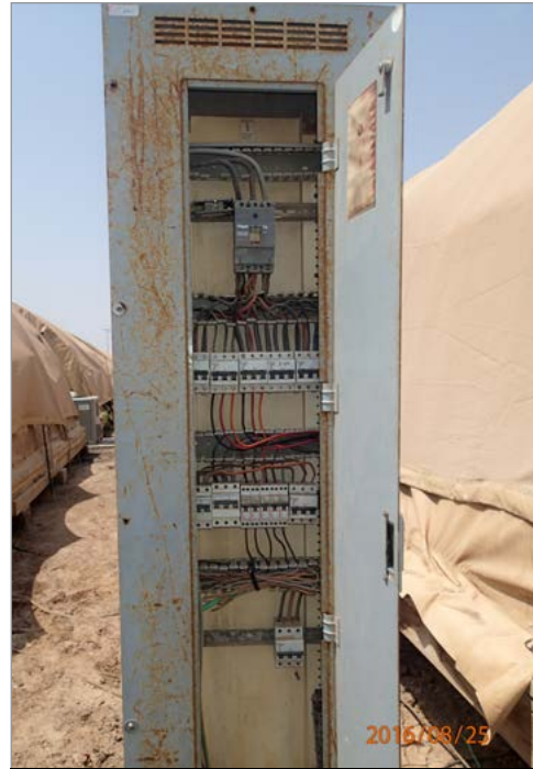
Figure 2. Electrical panel environmental degradation (Deficiency No. CLD-EL-160902-020)
