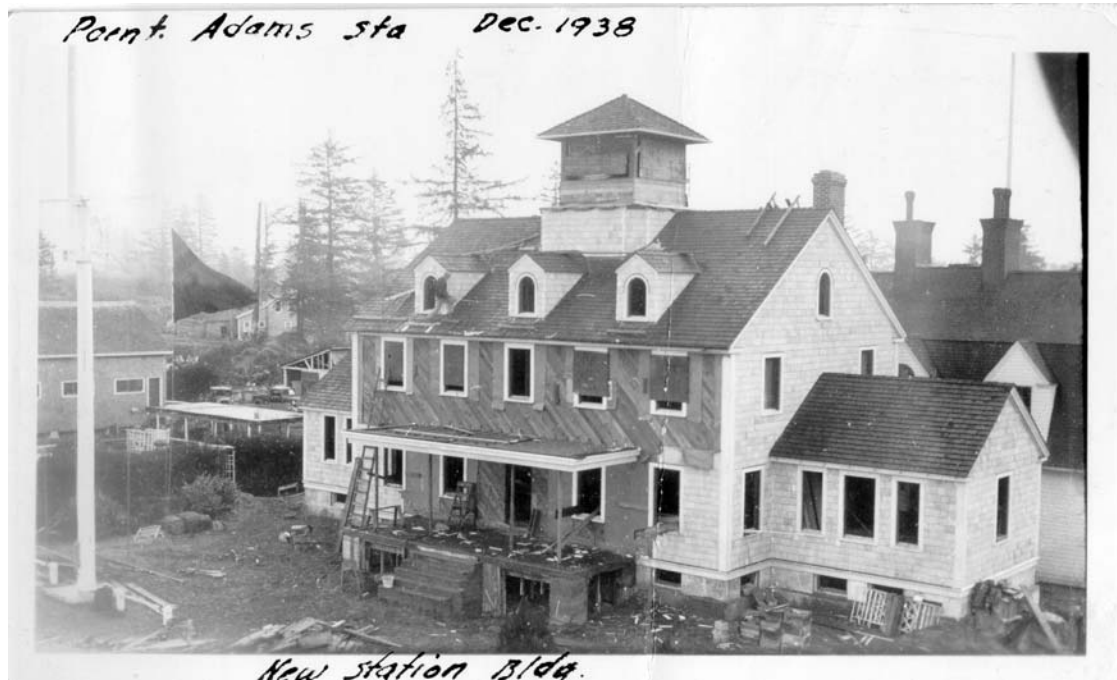
"Point Adams Sta. Dec. 1938. New Station Bldg." Stamped on back of photo: "Office Div. Civil Engineer, Seattle Div. Dec 28 1938." No other information noted.
