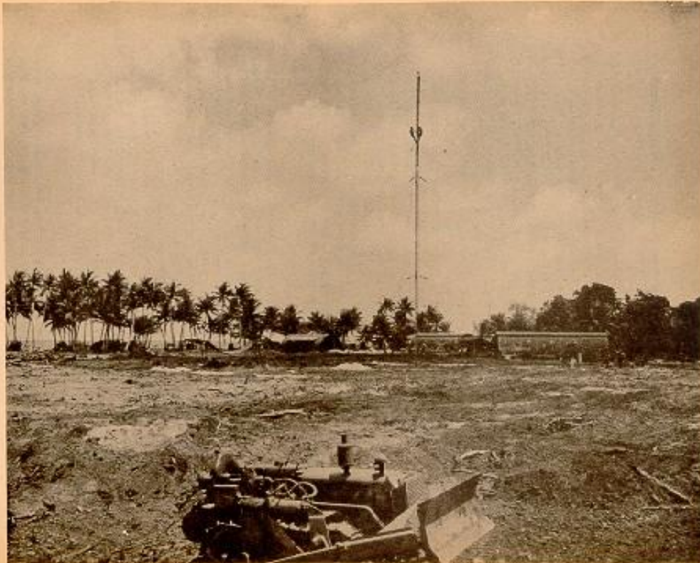
CLEARING, VERTICAL RADIATOR, AND HUTS, KWAJALEIN
