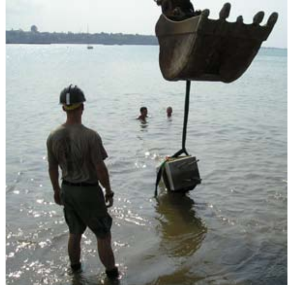
EA1 (SCW/DV) Christopher Munch (foreground) directs the placement of a grade beam while BU2 (SCW/DV) Joshua Sisson (rear left) and SW1 (SCW/DV) Anthony Wright wait at a safe distance to check its resting position underwater.
