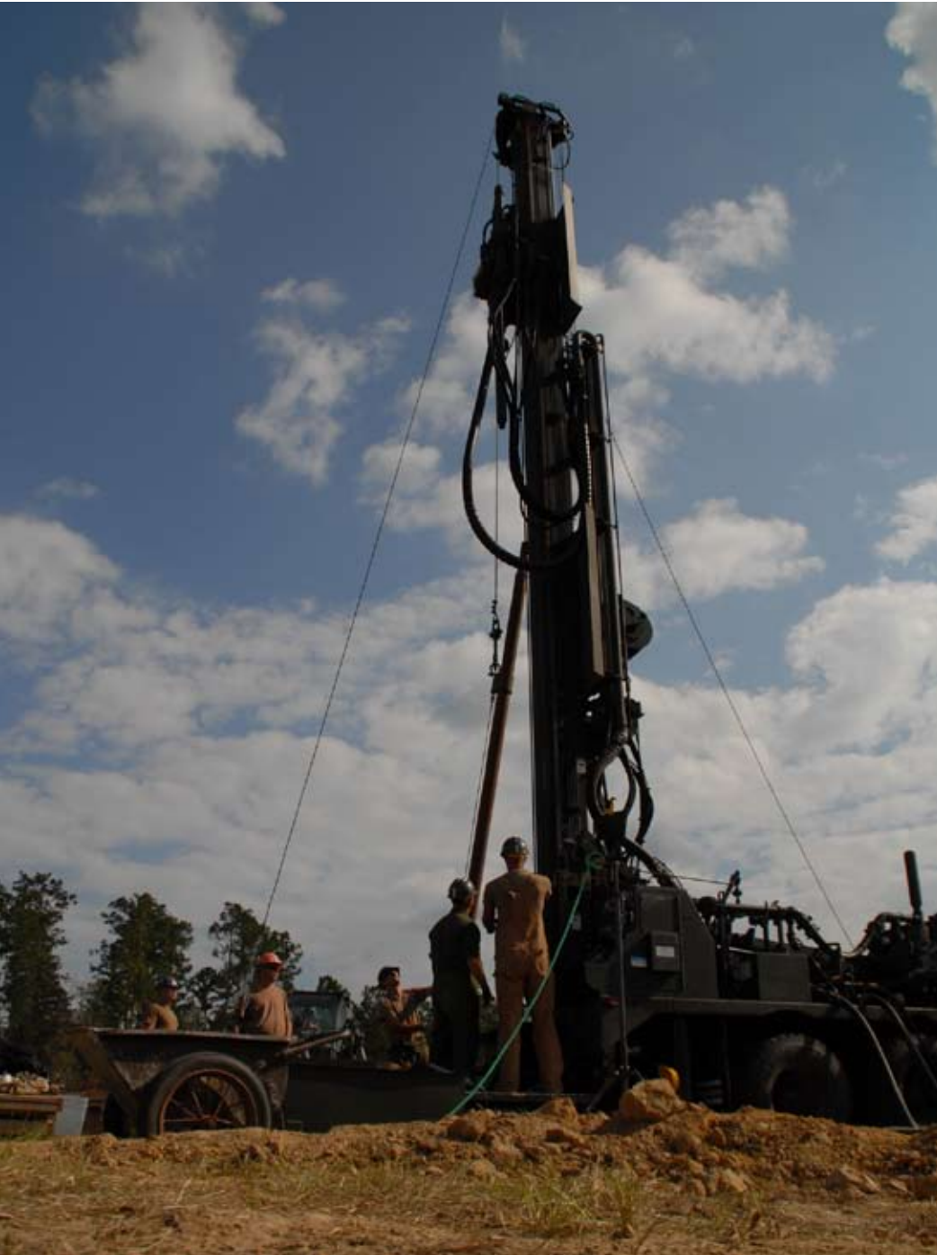
Seabees attached to NMCB 74's water well detail drill a 200-foot hole with an Atlas COPCO T2W at Camp Shelby, Miss., in mid-October.
