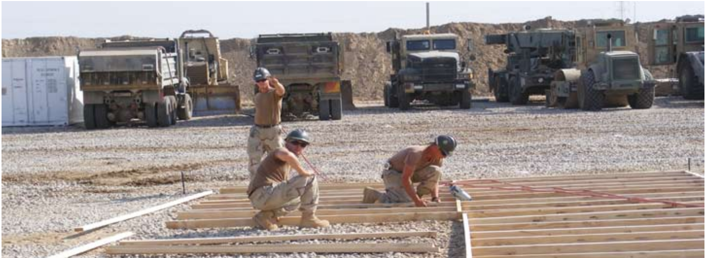
(Left to right) BU2 Steven Laucher, EO1 Mike Turton and BU2 Doug Shaner, ACB 2, build a deck for one of 14 MGPTS Large tents at Checkpoint 4 in the Wasit Province in Iraq.
