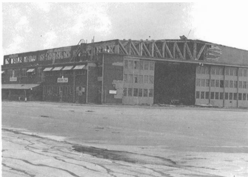
Hurricane damage, Homestead Army Airfield, September 1945
